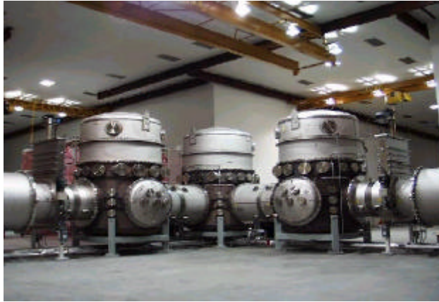
Figure 19. A photograph of the large vacuum chambers containing the various LIGO detector components is shown. These chambers are isolated from the long vacuum pipes by gate valves to access the equipment.
