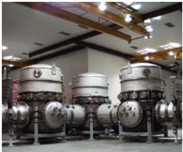
Figure 3 LLO vacuum equipment
